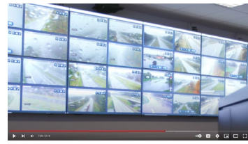
Traffic Operations Center/ Customer Service Center
